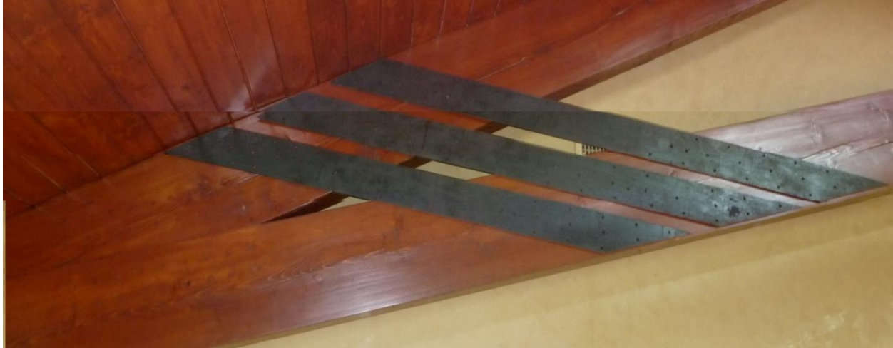
Straps on repaired scissor truss – basically, the aspect ratio of this plate and its connectors makes it behave more like a single axial strap (or, even, akin to a fully-threaded screw)
